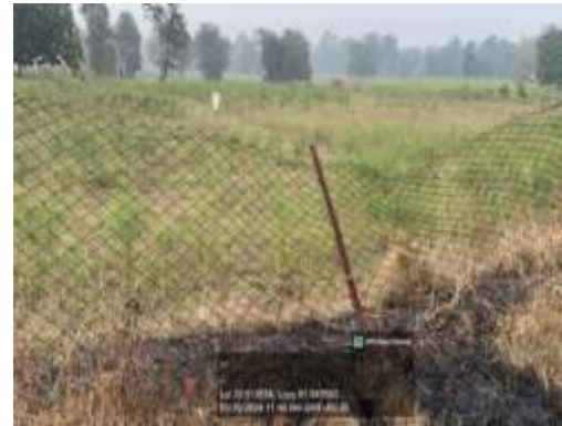
Fence damage by Elephants, Magdhi Range, BTR
